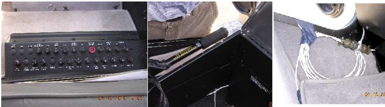
Figure B.2: Power Cable Routing: CB panel, under seat, cable dressing.
